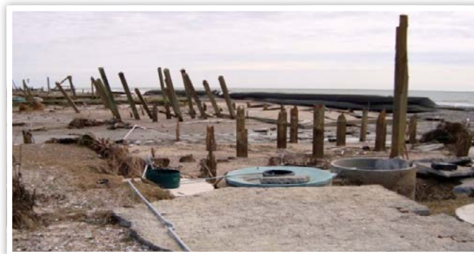
Elevating his home above the Hurricane Ike storm surge saved the house of this Galveston County home owner (FEMA photo).
